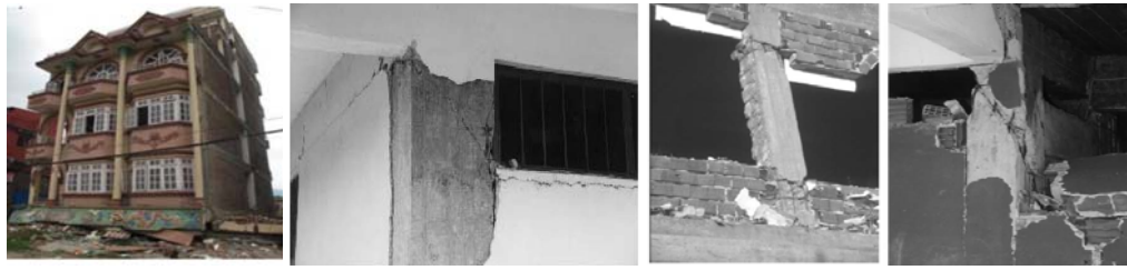
Figure 3: (a) Soft story failure; (b) Short column effect due to window opening; (c) and (d) Short column effect due to partial height of masonry infill wall [8]
